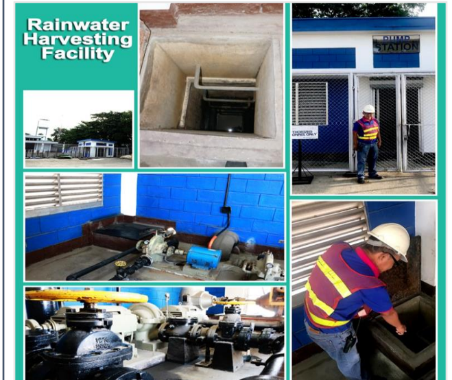
Constructed Rainwater Harvesting Facility
